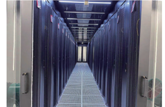
GDS Data Center
